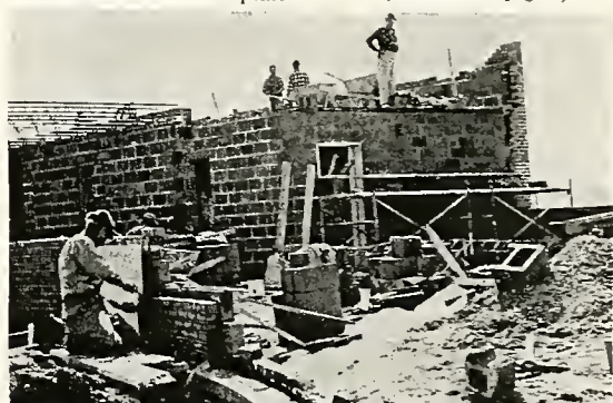
Sutton hill has been transformed into a hub of activity as work crews erect the new womens residence hall which is to open doors to 188 women September 1.
