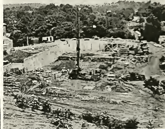
CONSTRUCTION GOES ON -- The new chapel continues to go up and the beams get higher and higher. The chapel is due for completion in the summer of 1966.
