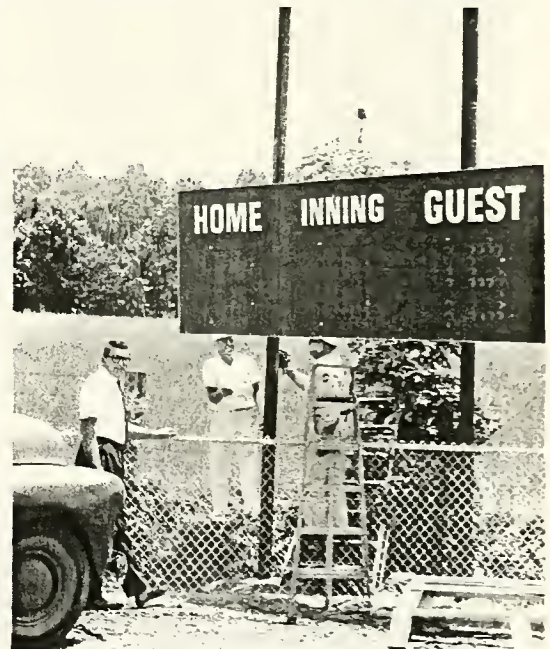
NEW ADDITION -- Coach Stout helps (7) to put up the new scoreboard on Anglin Field.
