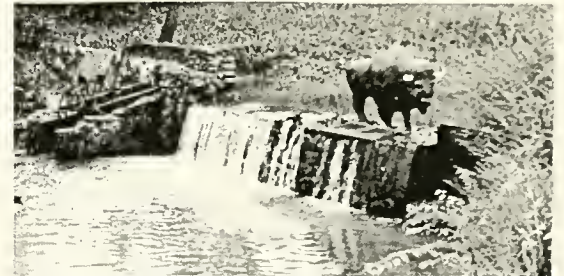
Maintenance work on the banks of Buffalo Creek continues as the water wheel was restored. The gazebo, whose foundation can be seen in the upper-right hand corner of the photo, is presently being constructed. The railing for the gazebo can be seen in the middle of the dam. (Photo by Tim Kirk)
