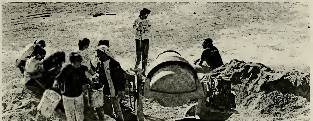
Students mix concrete for a driveway at Casa Hogar, the children's home run by Vida Nueva ministries in Piedras Negras, Mexico. Photo by Lance Risinger.
