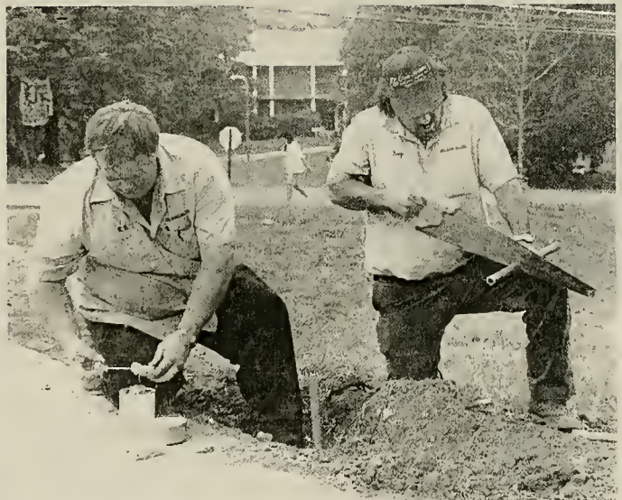
Milligan maintenance lays fiber optic cable next to the road up Sutton Hill. Photo by Barbara Allen.
