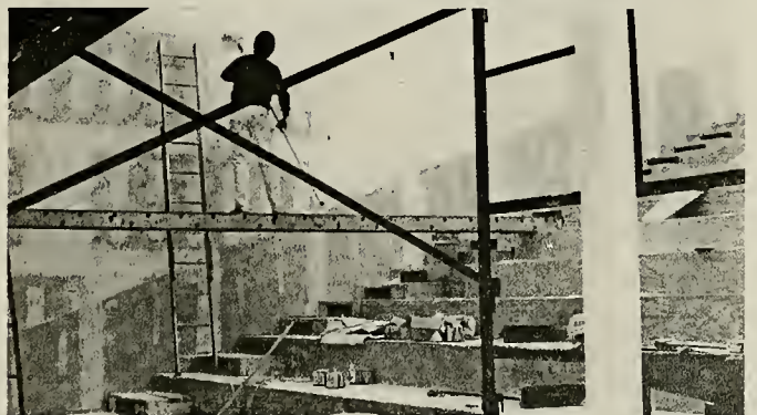
Construction is well underway for the 144-seat Wilson Auditorium in Hardin Hall. Photo by Kip Lines.
