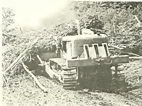
FIELD HOUSE PROGRESSES -- Due to unforeseen difficulties, Tennessee rain and Tennessee dirt, construction of the field house has been delayed.
