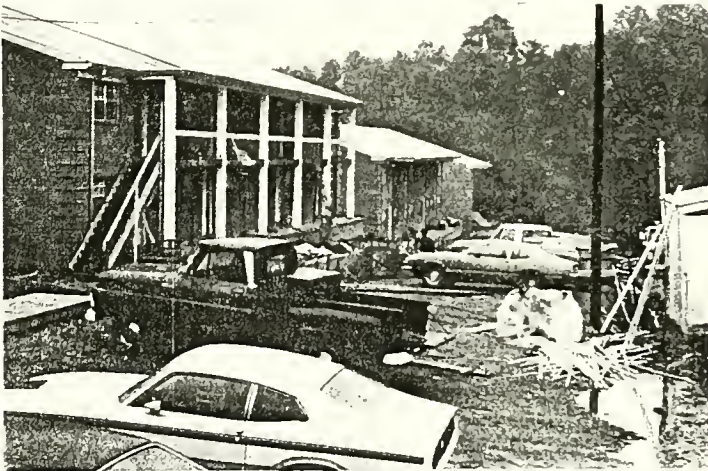
TAKING SHAPE -- Haphazard conditions prevail as the married student housing complex meanders toward completion. Delays in construction have caused both financial and convenience problems for prospective residents. (See related article, page 4)
