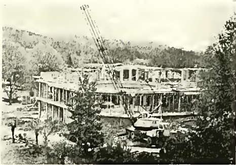
SIGNIFICANT PROGRESS — Daily progress on the external construction of Milligan's Science Building can readily be seen. Despite recent generous gifts to the college, funds are still needed for the completion of this building.
