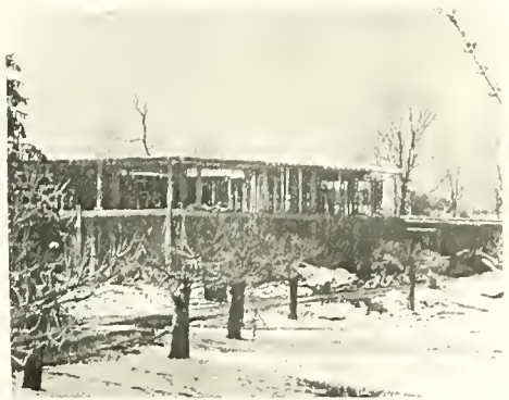
SCIENCE BUILDING -- Construction continues on Milligan's new science building, which should be in use by next fall.
