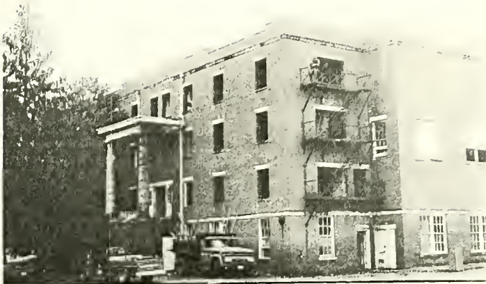
Cheek Hall is in the process of being demolished. The resulting space will be used for parking.
