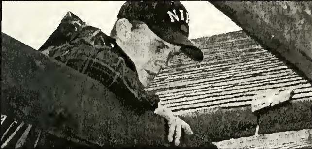
2002 Milligan graduate David Mayer builds a roof as part of last Saturday's Habitat for Humanity project at Appalachian Christian Camp. This was the group's second work day.
