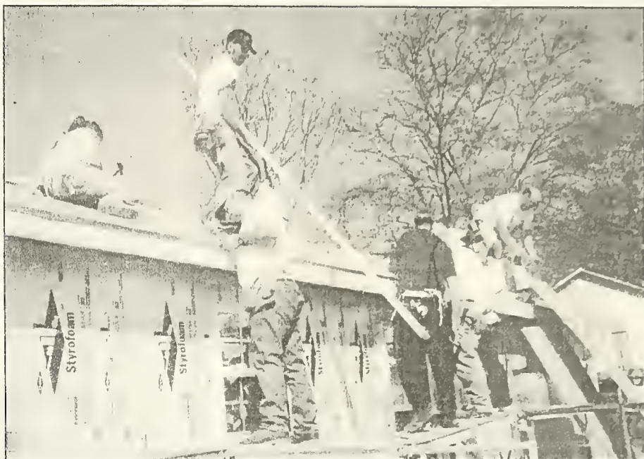
Milligan Habitat for Humanity students cooperate with a group from Illinois to build a three-bedroom house in LaGrange, Ga. on the site of a future Jimmy Carter workcamp.
