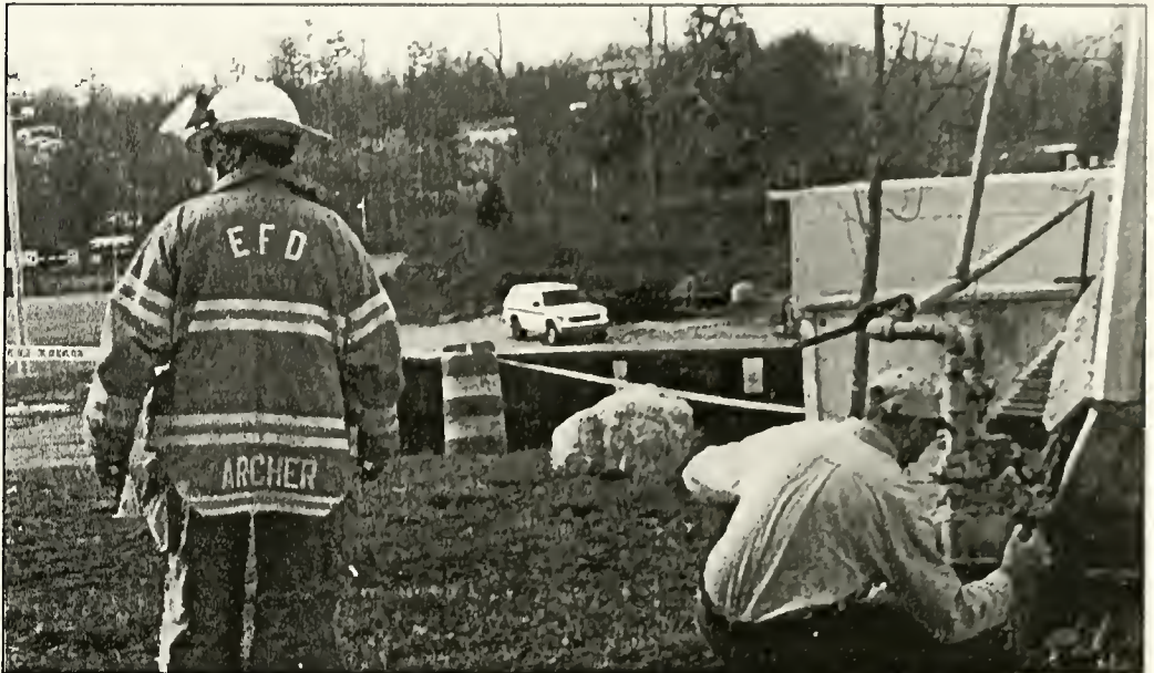
On Saturday, workers disconnected the gas from the left side of the physical plant for safety purposes. This side of the building had shifted off its foundation and leaned towards the center. -Photo by Jennifer Soucie
