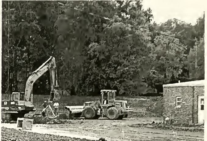
Work crews prep the area surrounding FOB in preparation of new education center.
