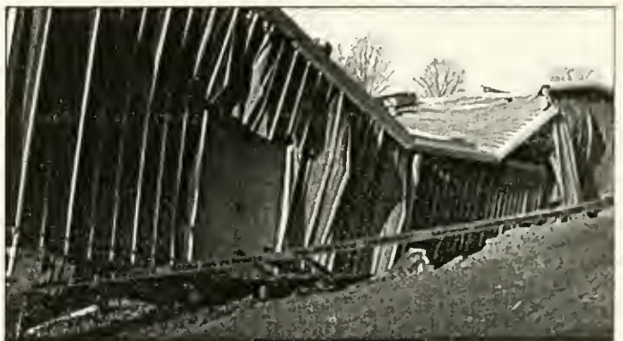
The gravel area was the parking lot in front of the physical plant, which makes a steep drop. Standing from the edge, contents of both the attic and basement are visible. -Photo by Jennifer Soucie
